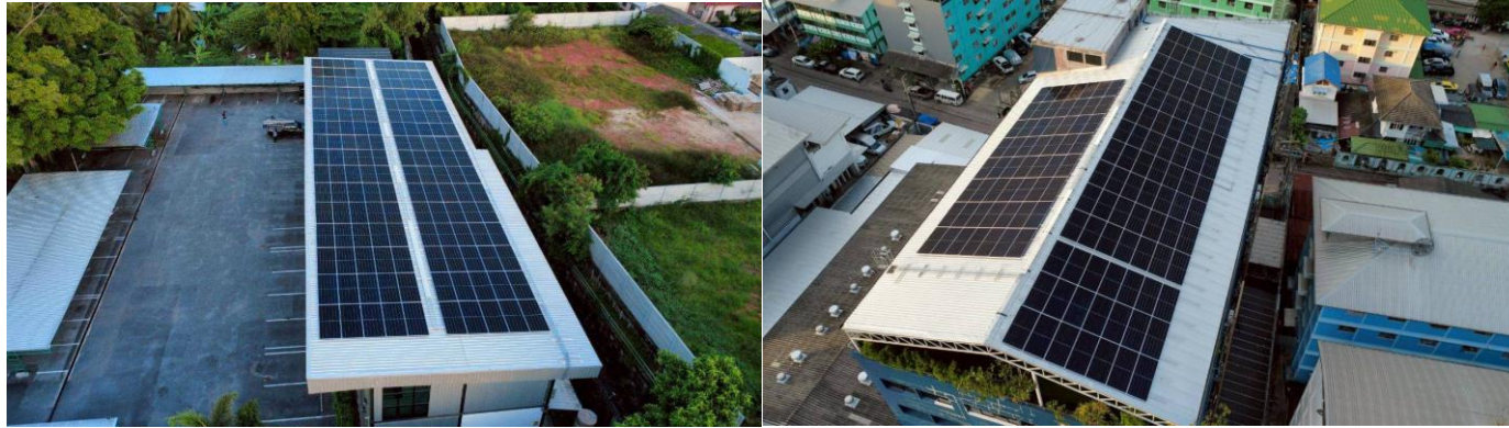
Solar Rooftop at the Headquarters
